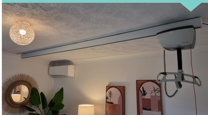
Straight track with power traverse motor.
